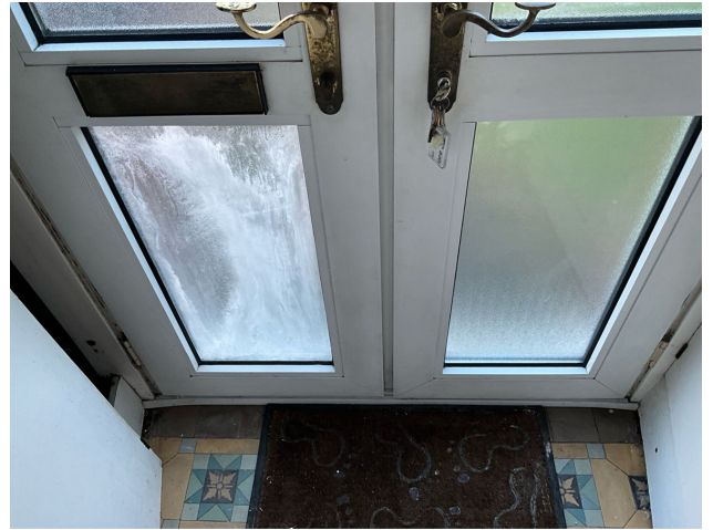
Failed glazing, safety glass?
