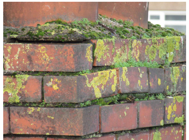
Loose material, uneven brickwork.
