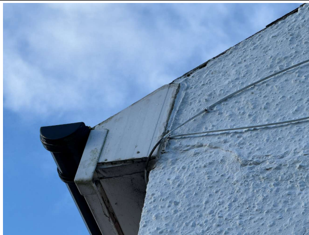
Poor fitting at rear.
