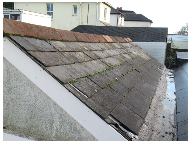
Also note gap where tile missing.
