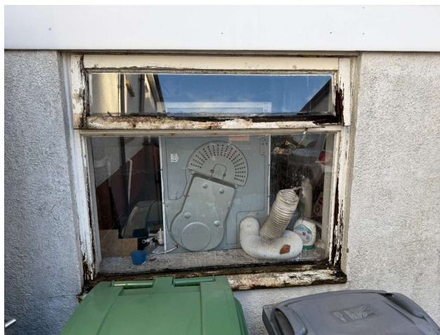
No safety glass, rot.
