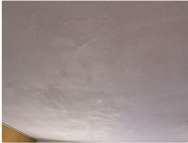
Note cracking and textured finish.
